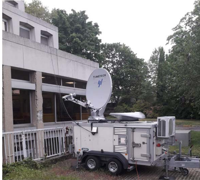
Figure 6-12: View of the mobile station at OP
