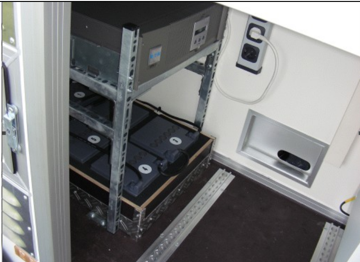
Picture 6-5: UPS and Batteries
