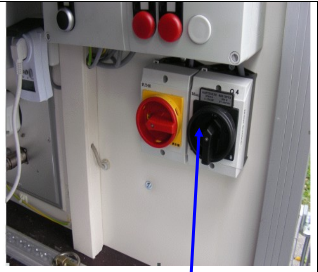
Picture 6-6: Mains Switch
