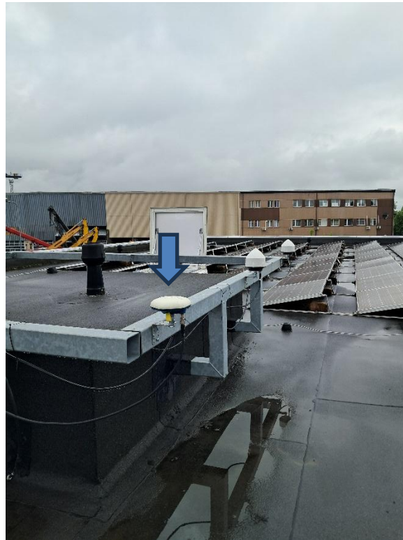
Figure 3-5 The PTBM antenna installed at Metroserf. The blue arrow points towards the PTBM antenna. The EE01 and EE02 antennas can be seen in the background.
