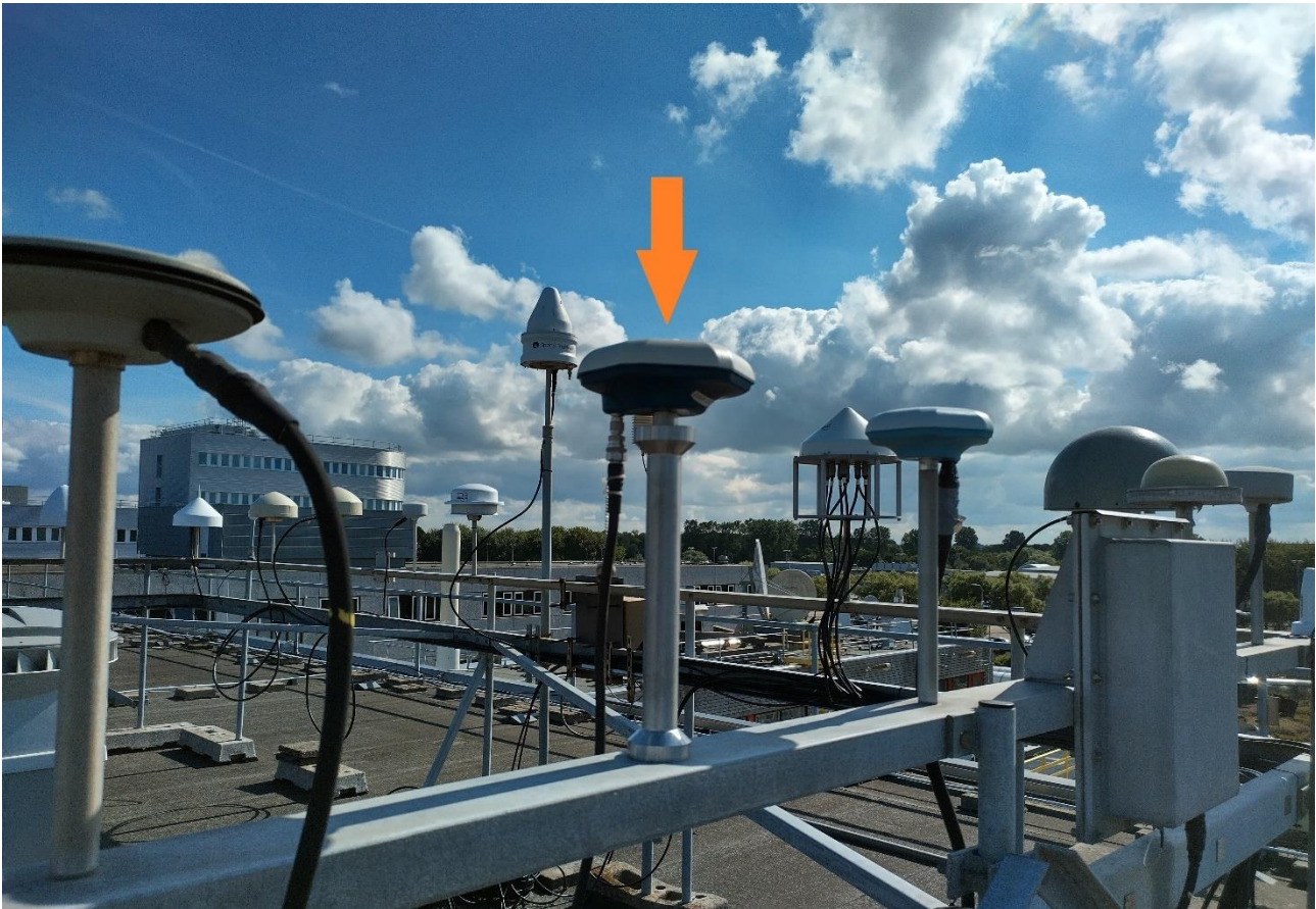
Figure 3-5 Antenna installation on the roof of the CK building at ESTEC, the arrow pointing to the PTBM-antenna
