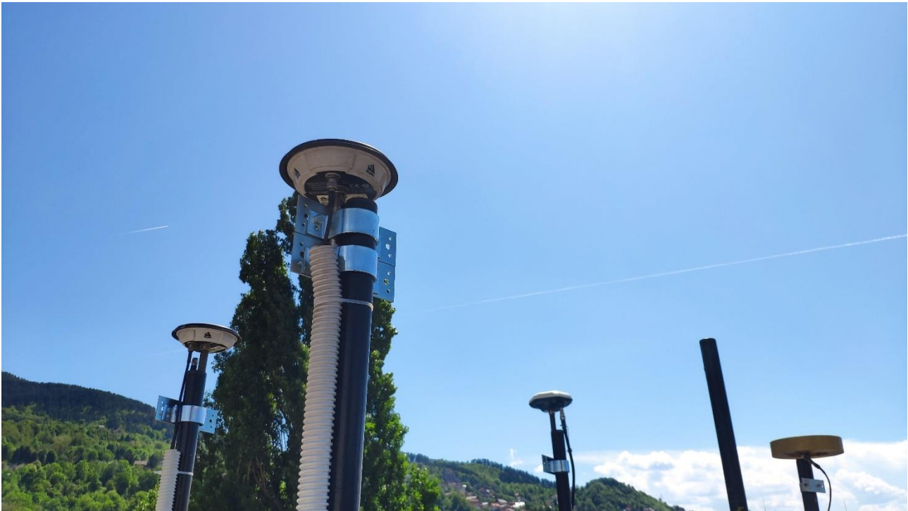
Figure 6-2 Antenna installation on the roof of the IMBH building (PTBM background, middle)
