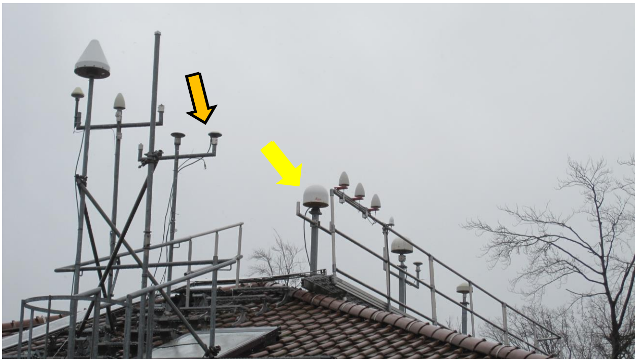
Figure 4-4 Installation of GNSS antennas at PTB, PT13 antenna (yellow) and PTBM antenna during CC1 and CC2 (orange)
