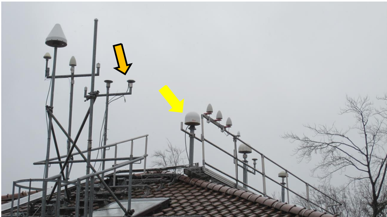
Figure 4-3 Installation of GNSS antennas at PTB, PT13 antenna (yellow) and PTBT antenna during CC1 and CC2 (orange)
