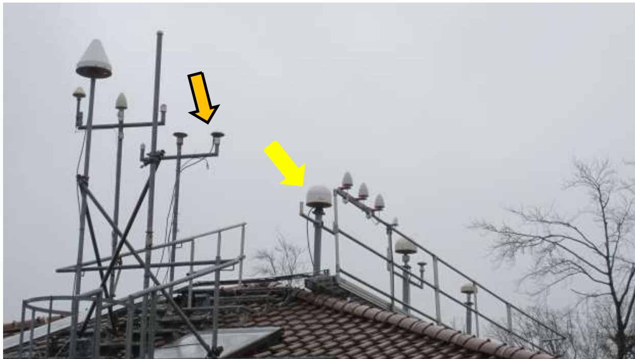
Figure 4-5: Installation of GNSS antennas at PTB, PT13 antenna (yellow) and PTBM antenna during CC1 and CC2 (orange)
