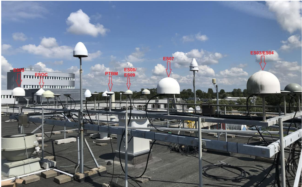
Figure 6-2: GNSS antennas on the rooftop of a building at ESTEC hosting the time laboratory
