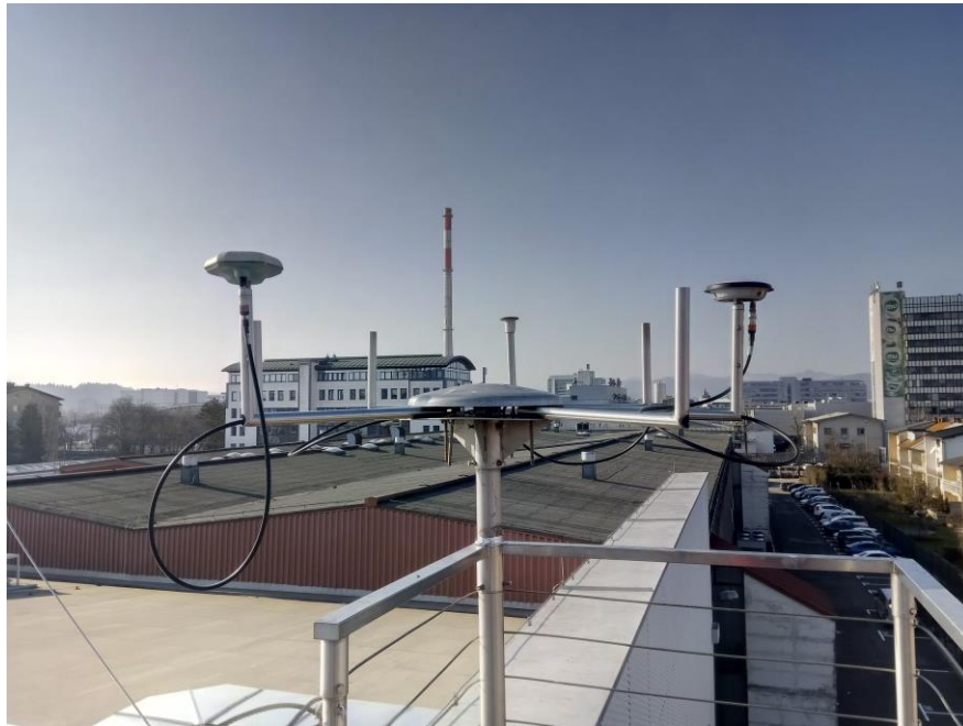
Figure 7-2 Antenna installations on the rooftop of the SIQ building
