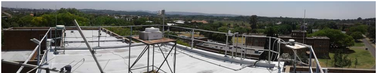
Figure 6-2: Antenna position on the rooftop of the NMISA building and panoramic view of the antenna installations (lower image)
