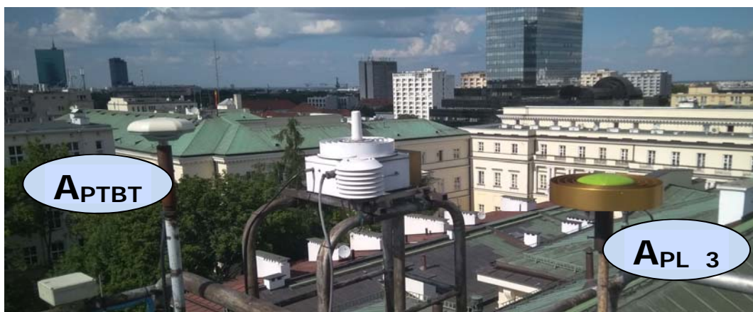
Figure 7-2 Mounting of GNSS antennas on the roof of GUM during data taking:PTBT antenna (left), PL_3 antenna (right) and TTS-2 antenna (middle)
