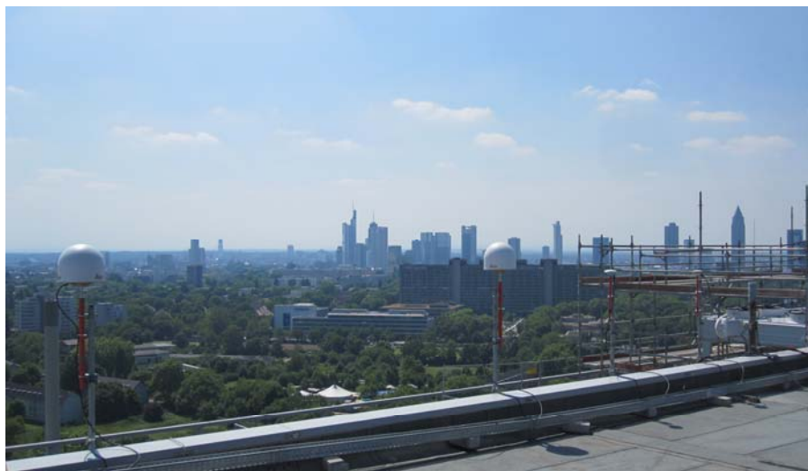
Figure 6-2: Antenna installation on the rooftop of the DTAG building: Horst Ender fixing the PTBT antenne (3G+C), and the two DTAG Leica AR25
