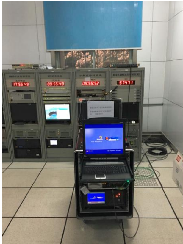
Figure 4. Calibrator installed in NTSC
