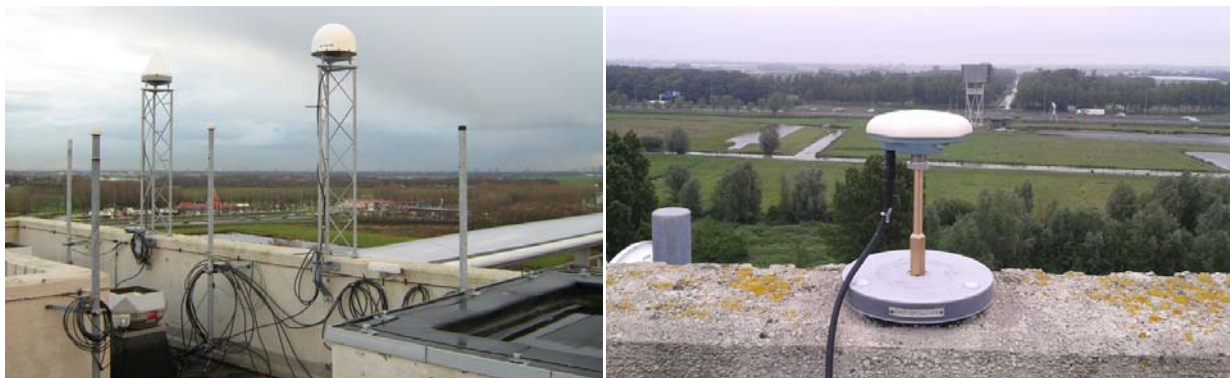
Figure 8-2: Installation of GNSS antennas on the VSL roof: from left to right: VSLG, VSLF, and PTBT
