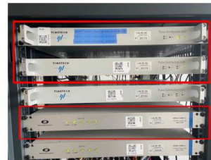
UTC(IT) TF signals at RadioNavigation Lab. To GNSS receivers (TimeTech Pulse Distribution Unit and SDI HPDA-15RM-C)
